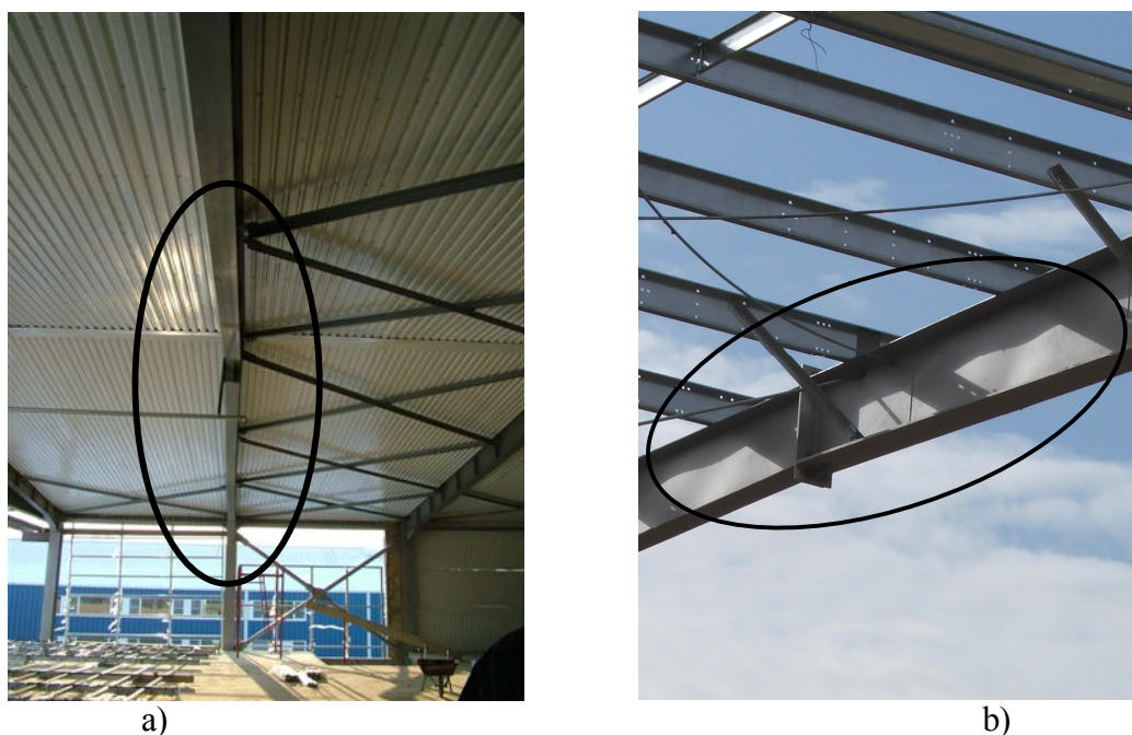
Figure 1. Imperfections recorded on site: a) erection imperfection (er); b) manufacturing imperfection (man).
