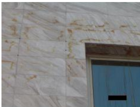
Picture 2. Degradation of exterior plates [3]
