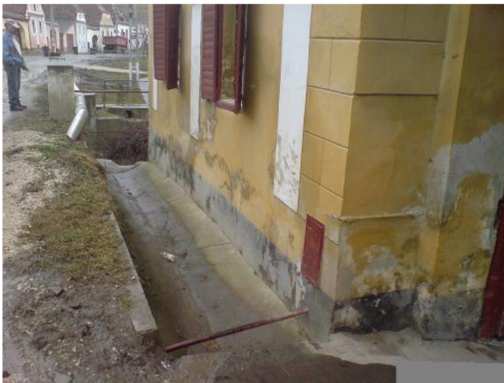
Picture 4. Degradations due to dampness
