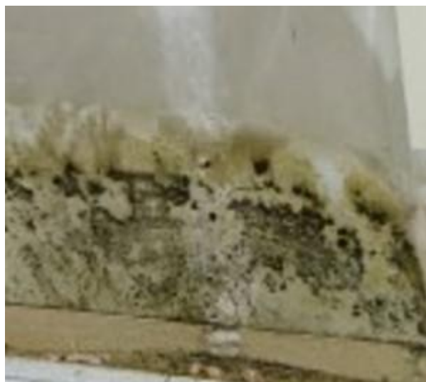
Picture 5. Degradations due to mold
