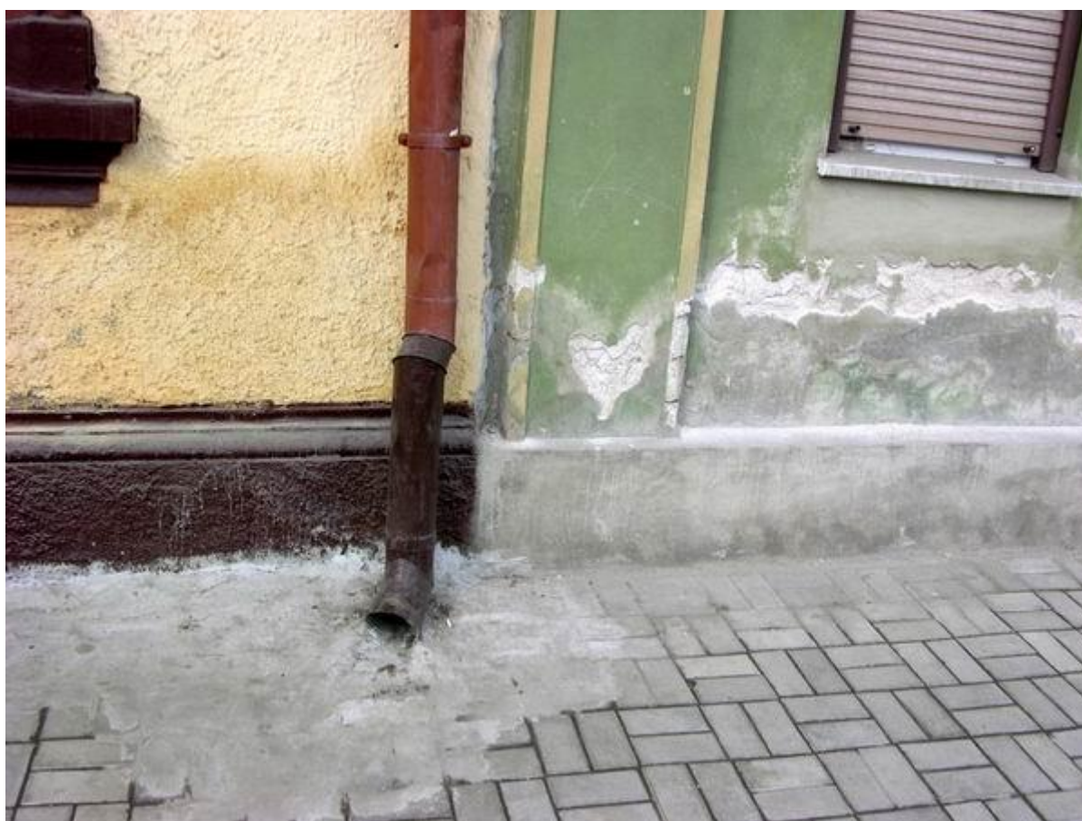
Picture 3. Degradations due to rainwater and salts [3]
