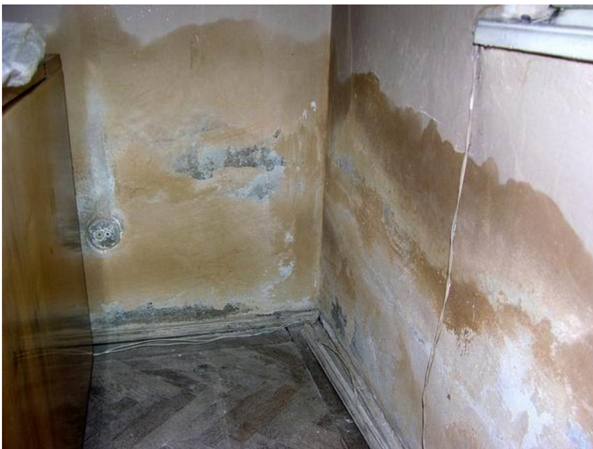
Picture1. Deterioration of painting [3]
