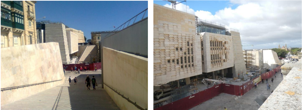
Fig . 62, 63 The construction site – April 2014 [Source Fig 62 and Fig 63: pictures taken by the author]
