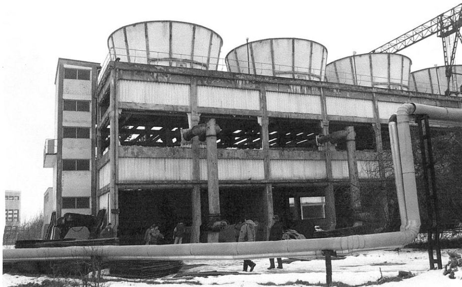
Fig.1. Forced draught cooling tower no. 1. General view.
